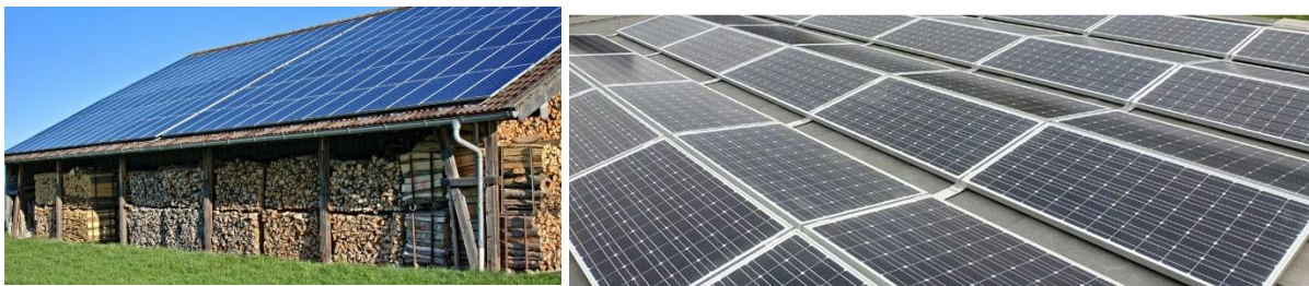
Figure 1, 2 - Multiple fire risk and a flat roof with full of solar panels
