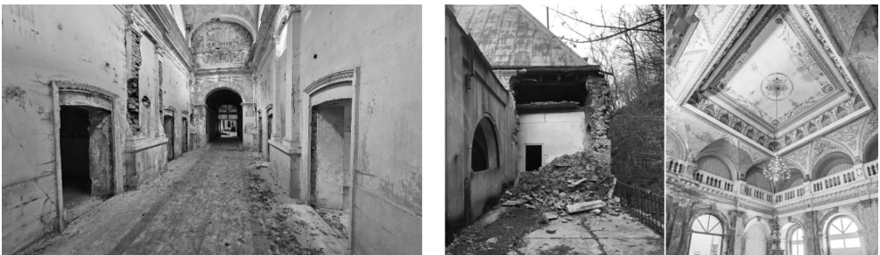
Figure 5. Băile Neptun degradation situation
